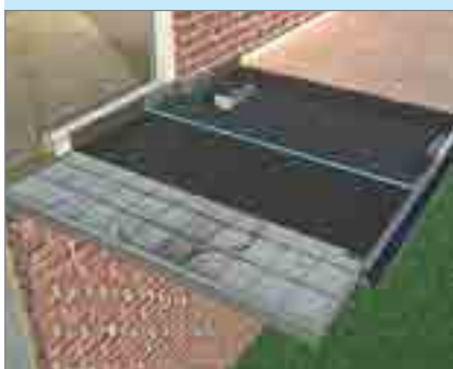
Substructures in need of renovation
